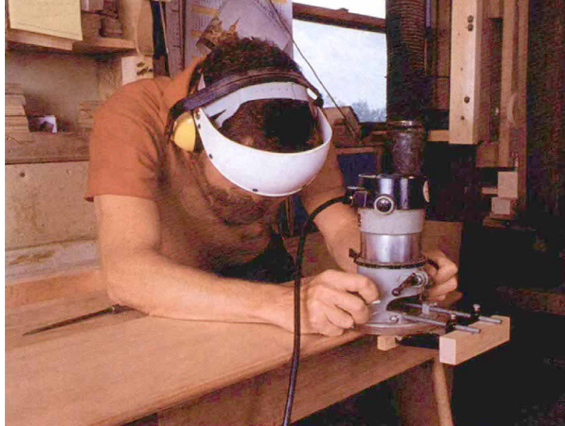
To ensure proper hinge placement, Campbell uses a fence when routing the hinge mortises.
